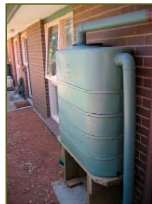
Rainwater collection system
