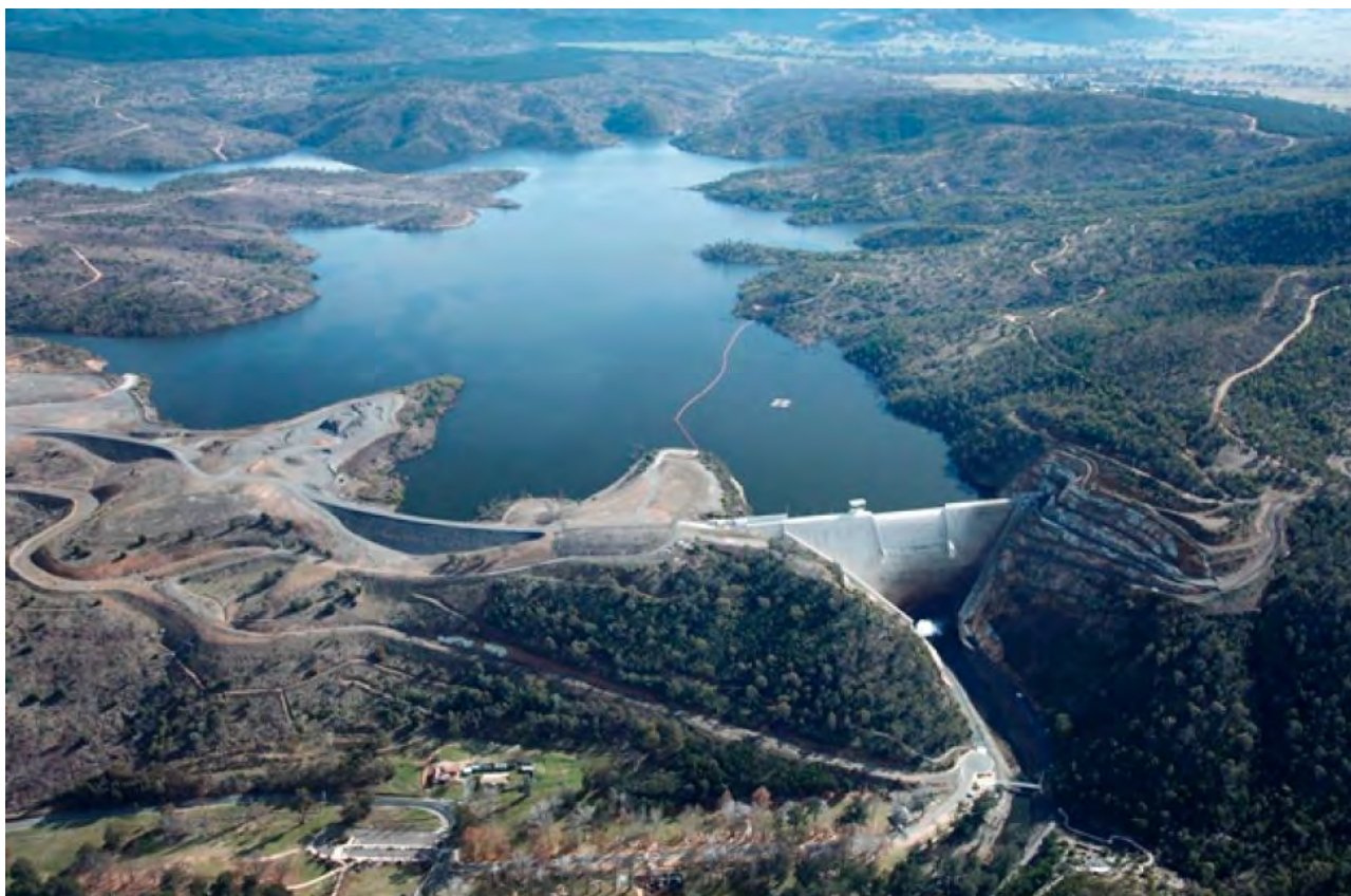
Aerial view of new Cotter Dam wall under construction (EPSDD photo library)
